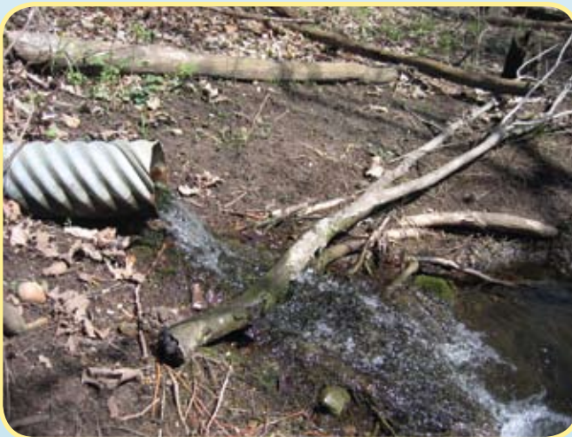
Figure 7 - Stormwater runoff entering a stream
